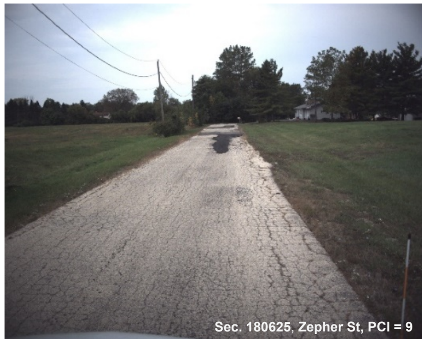
Figure 8: Sample pavement image with PCI value (Failed)
