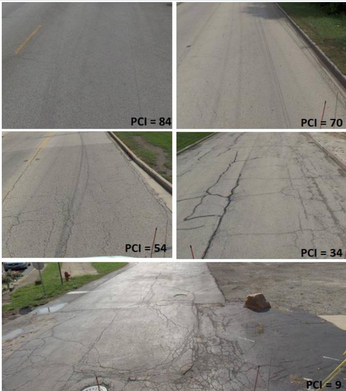
Figure 6. Sample Pavement Distress Images with Different PCI Values.
