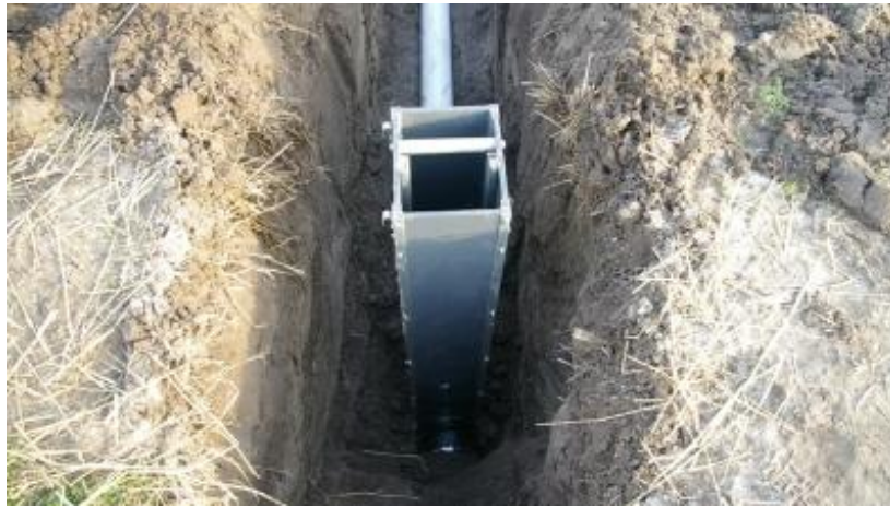
Figure 5-3. Image of control structure installed at tile outlet.
