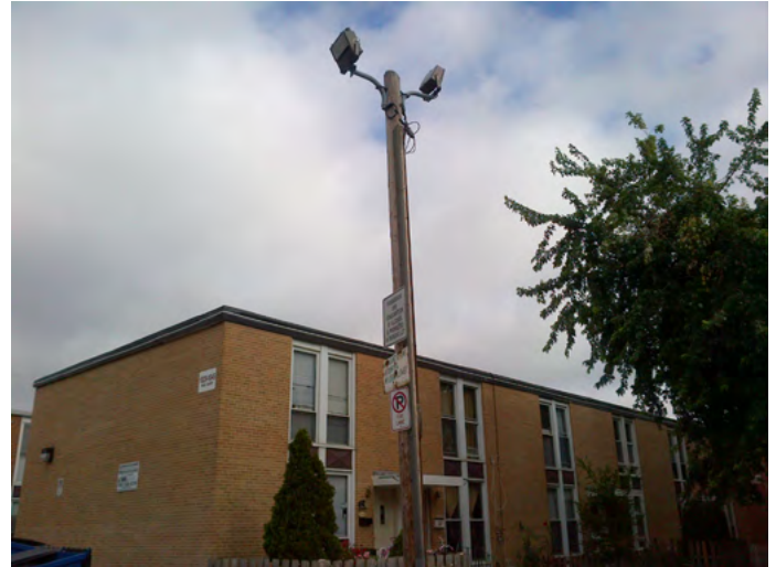
Figure 4.29: Pine Court’s courtyard is in need of additional lighting.
