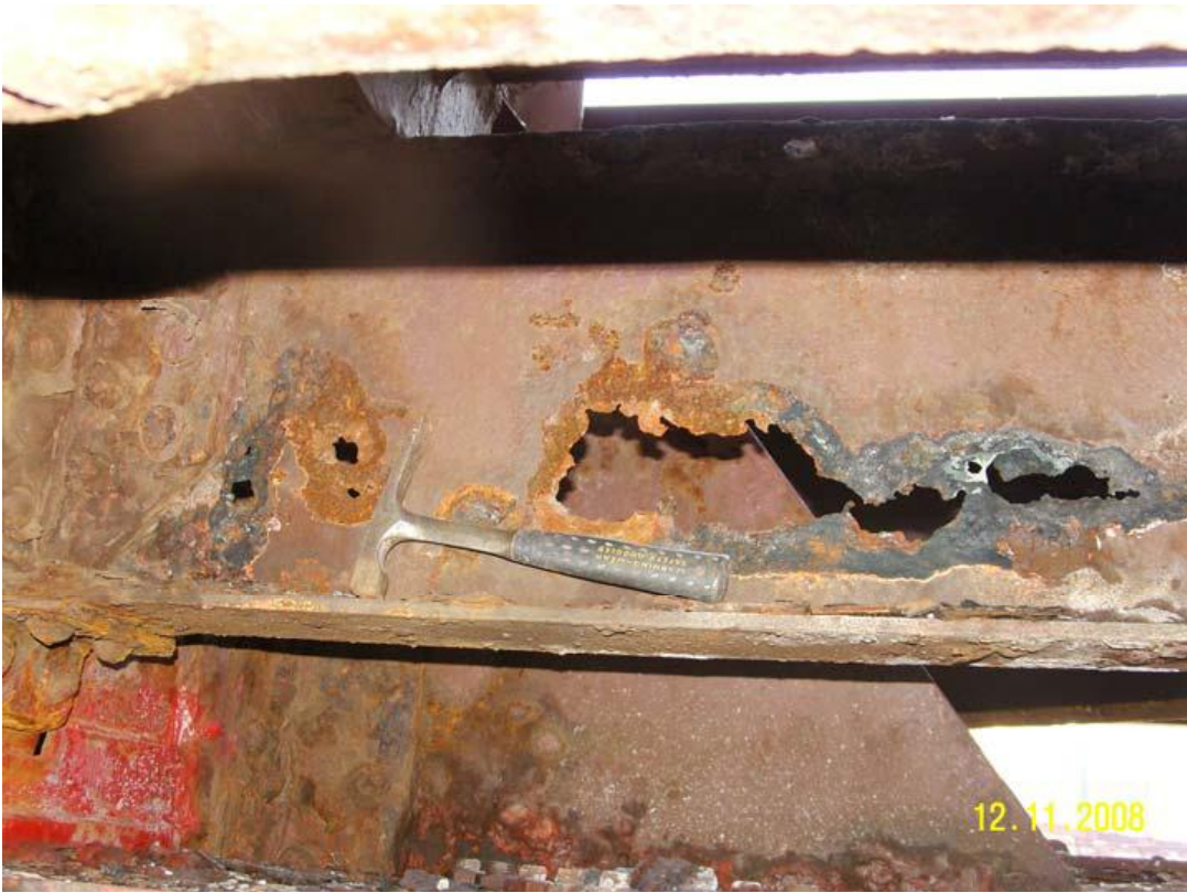
24" rusted web hole at north end.
