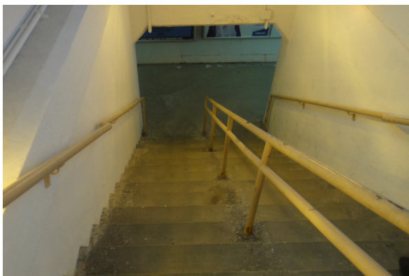
Olympia Fields Metra Station lacks ADA accessibility
