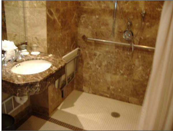
Lav obstructs transfer space at seat
