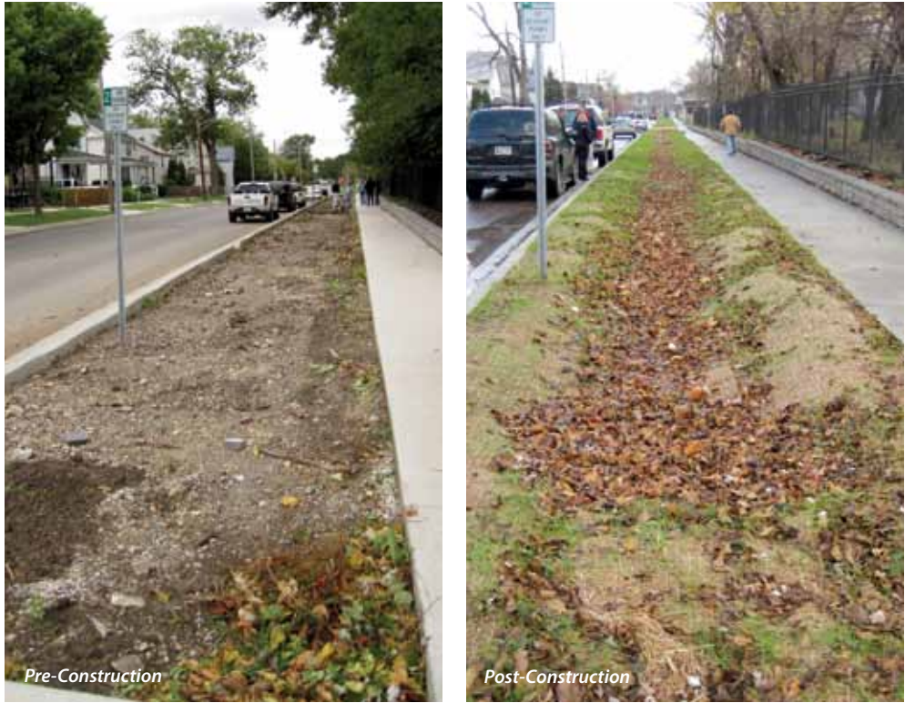
Decombination BMPs shall be designed to receive and treat urban runoff before it enters the Fox River. The project utilizes the right of way between the sidewalk and Spring Street (photos by H. Hudson and M. Elberts, CMAP).
