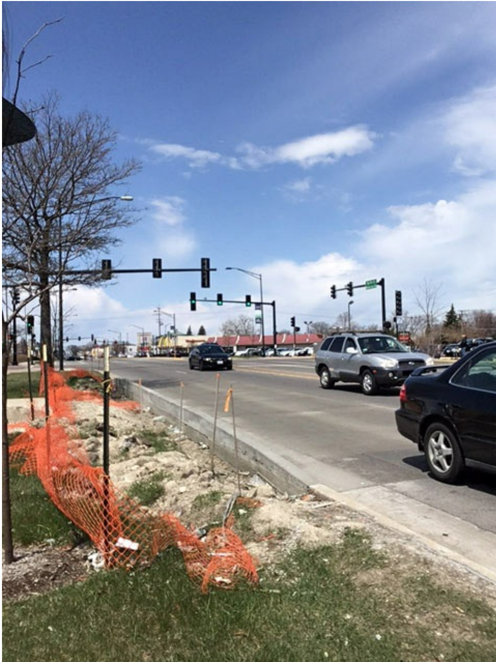
The location of future Pulse stations along Milwaukee Ave are apparent by the preliminary work already done. Photo by Jen Shea for The Bugle.
